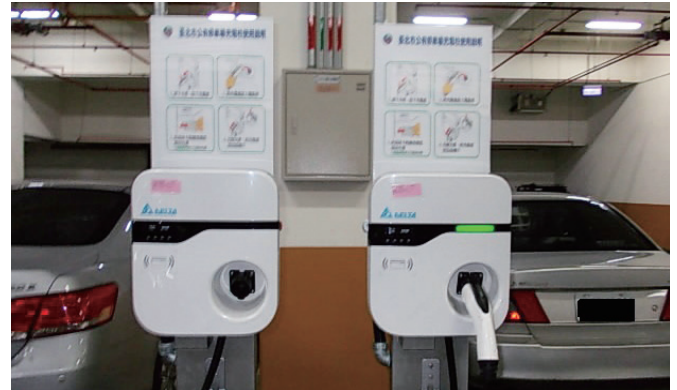
EV charging ports
