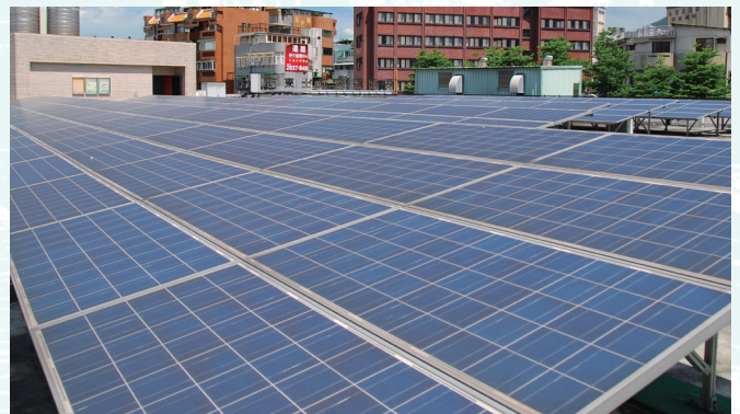
Solar PV system at Shidong Market
